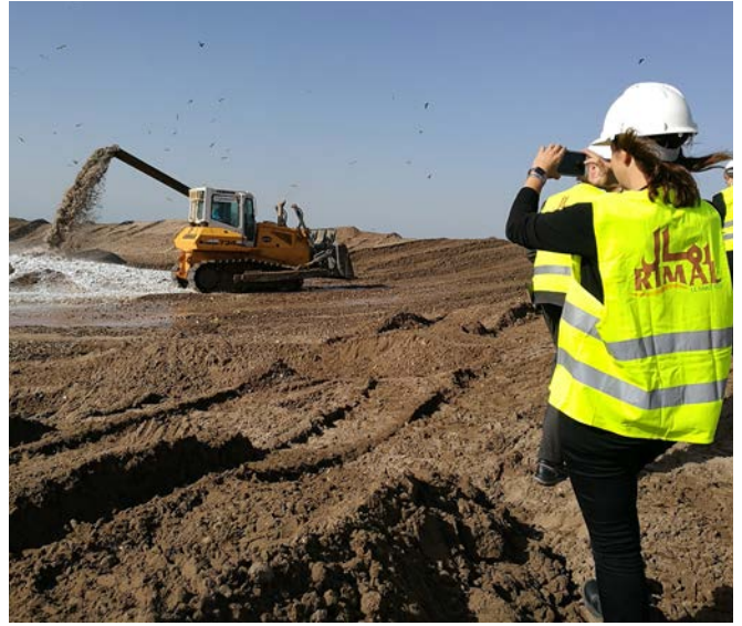
After the Board meeting, Drapor hosted a site visit to a sand mining site near the town of Azemour where the river Oum Rabia meets the ocean. The sand is used for construction purposes.
