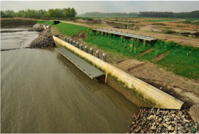
Figure 2: Sluices in the project area Kruibeke-Bazel-Rupelmonde
