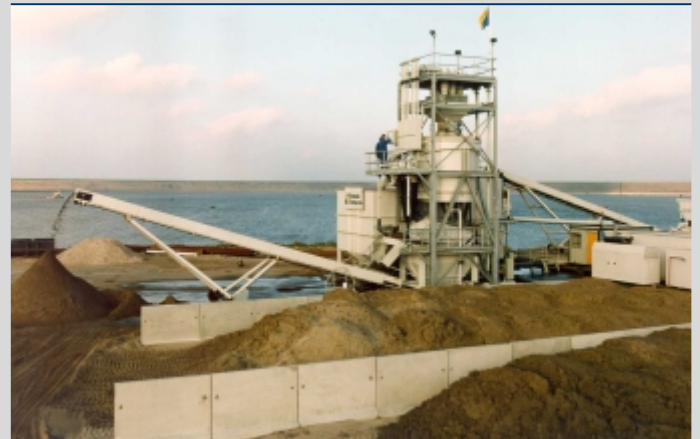
Hydrocyclone separation facility
