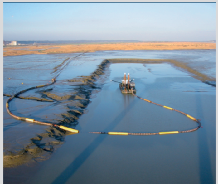
CSD with pipeline (source: Van Oord)
