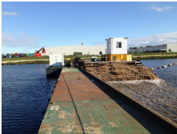
Figure 2: Project start – tricking thin layers of sand on the weak bottom of the former dredged material storage facility
