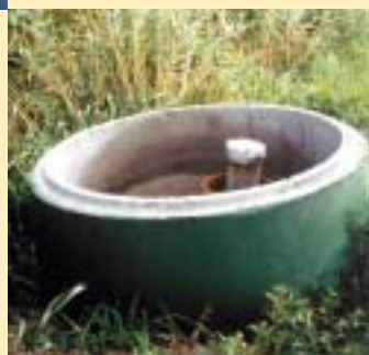
A monitoring well is used to test groundwater quality, in the vicinity of the Francop site.
